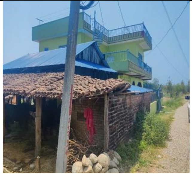
Figure 2: Affected part of load bearing shed of Rukmangat Ghimire, Chainage 2+340 – impact will be reconfirmed once final design is available.
